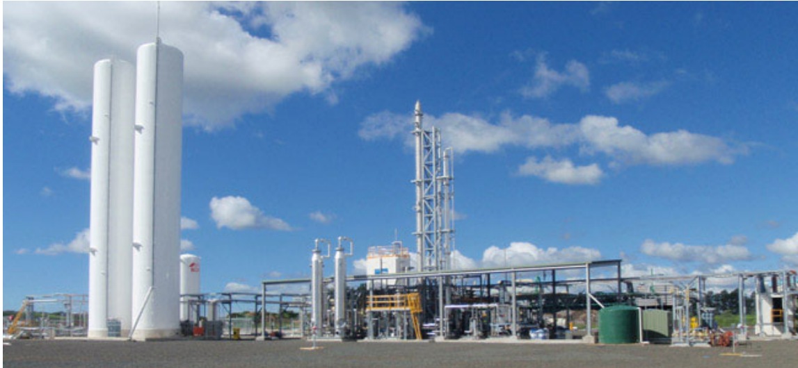
Figure 20. The BOC micro-LNG plant in Westbury, Tasmania.
